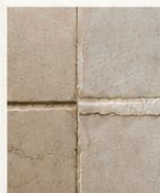
Uneven grout lines
